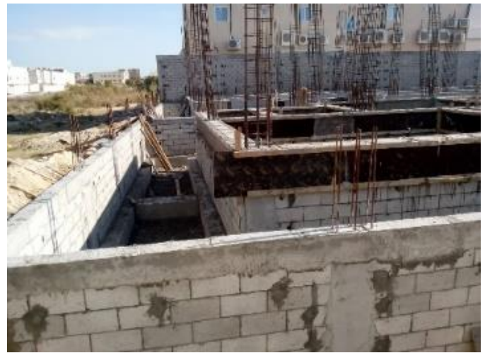
Figure2. Aldubaisi Fadhel house in Aljawharah, Tarout island, Qatif in process building, January 2019.
