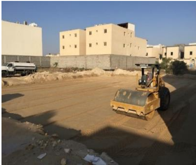
Figure 9. Aldubaisi Fadhel house in Aljawharah, Tarout island, Qatif. Under first stage process December, 2018
