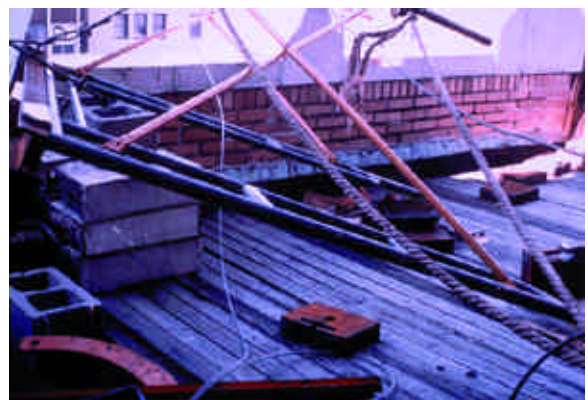
FIGURE 4.9 On top of the building above the decedent, a pulley device with counterweights had been knocked over by high winds. See next photo.
